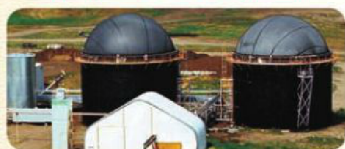
Anaerobic Digesters - Alberta, Canada
